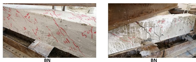
Figure 7. The Cracks Propagation in BN Beams
