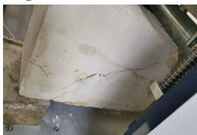
Figure 11. Beam B3 (I-section) Cracks
