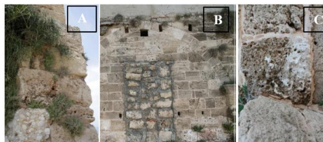
Figure 2: Images taken at site in Tyre City showing Structural and Physical Changes (Problems). (A): Spread of Plants; (B): Appearance of Cements sheets on main elevations; (C): Masonry and Stone Problems (appearance of Black colors, Bacteria, holes...) (Source: Author)
